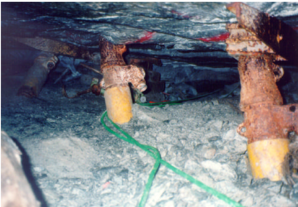
Figure 5.2 Problems result from poor control of props such as footwall punching when props are left in back areas and the inconsistent use of headboards.
