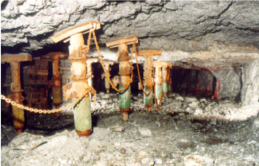
Figure 5.1 A proper prop control system will result in good working conditions with a cost effective support system.
