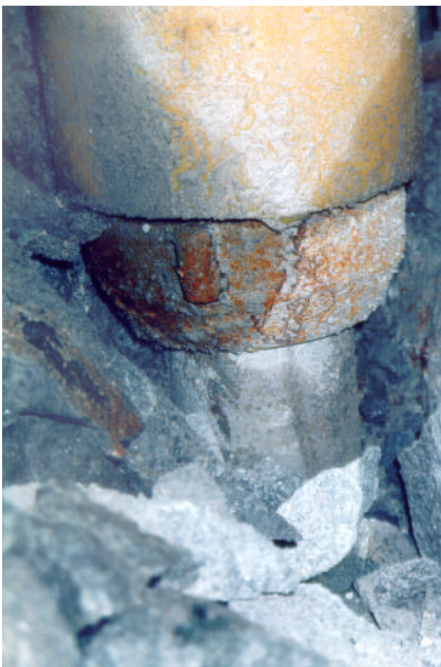
Figure 5.4 Footwall punching of prop in the course of normal stope convergence.
