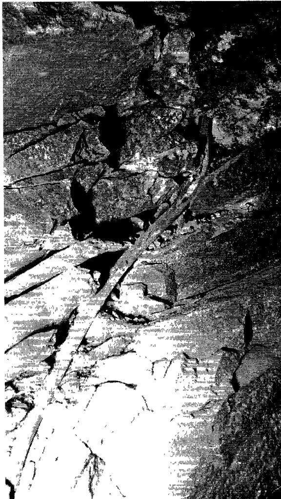
Photograph 4-2. Shear deformation of smooth bar rock bolt.
