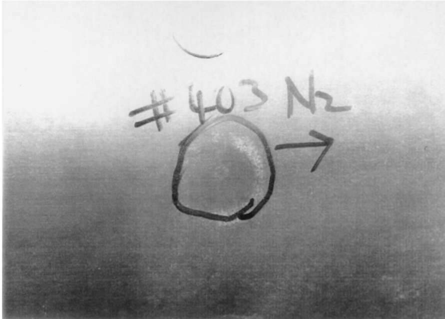
Fig. 3. A pimple defect, marked from factory in white but never repaired before pipelaying.
