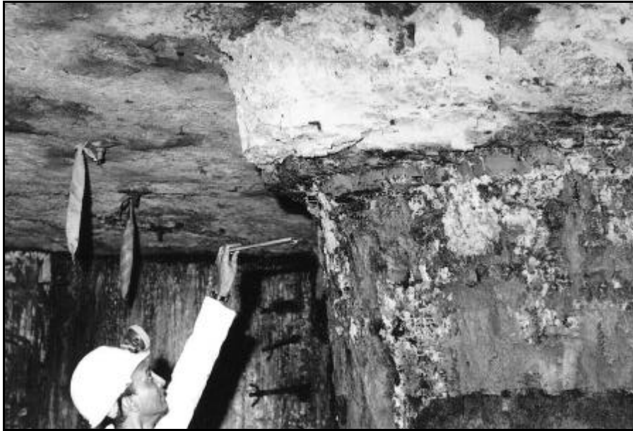
Figure A13: -Water leakage at top coal/roof contact
