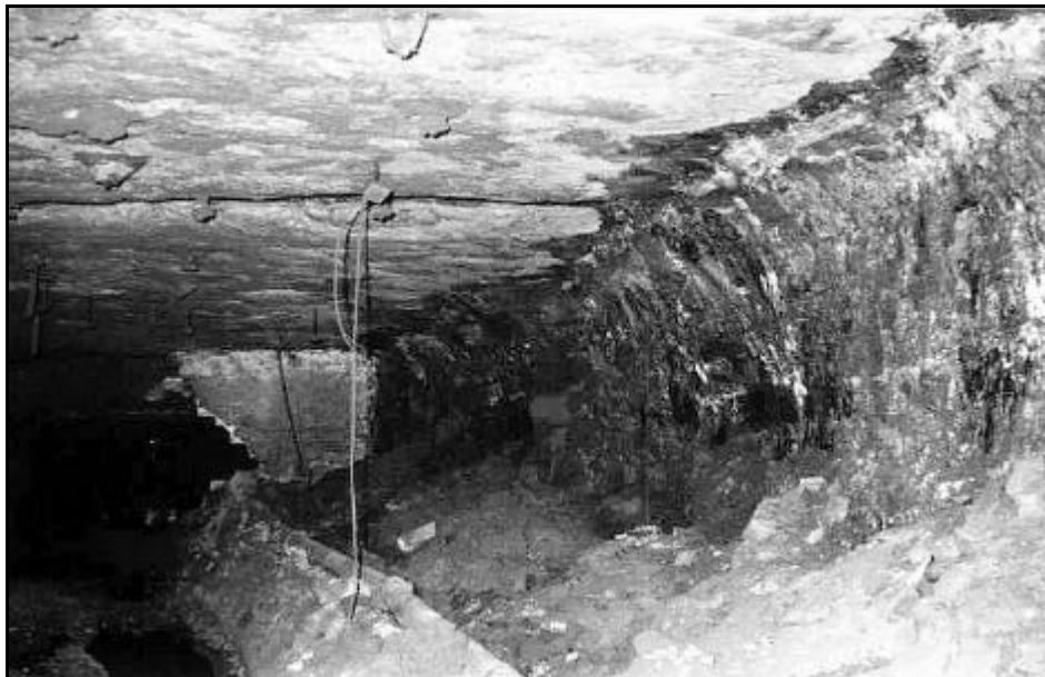
Figure A12: - Roadway side of the 50m wide barrier pillar demarcated for instrumentation
