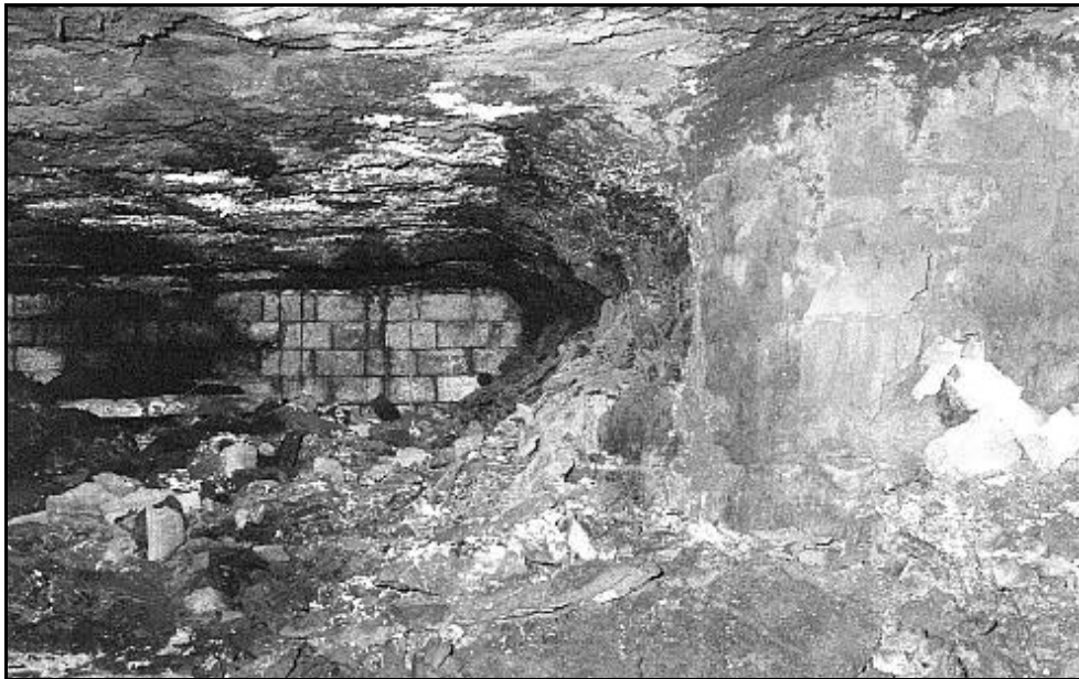
Figure A5: -Extent of sidewall spalling along barrier pillar
