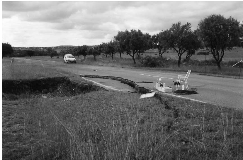
Fig. 6. Photograph showing the view from electrode position 19 and looking north over the bigger of the sinkholes in the direction of the start of the profile (position 1). Evidence of the smaller of the two holes (at electrode position 13) can be seen in the tree on the other side of the road that dropped vertically downwards so that its crown just protrudes above the ground.
