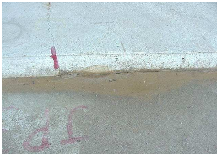
Figure 3. Pumping from under the leave slab, the right hand side of the crack
