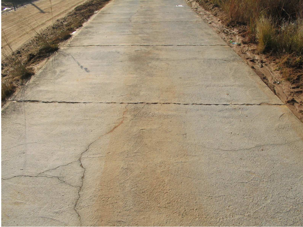
Figure 3. Typical cracks encountered on longer panels during the review of the sections. Note the good condition of shorter panels in the background.
