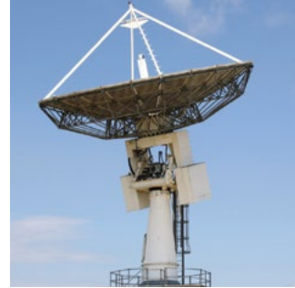
HBK-7: 13.2 m Ku/DBS-band antenna with a 2°/sec slew rate, programme and auto-tracking. Installed in 1998 for TOSS and IOT 4 support.
