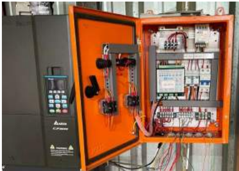
Figure 6: CP2000 Variable Frequency Drive and IIoT Unit Used in this Test.
