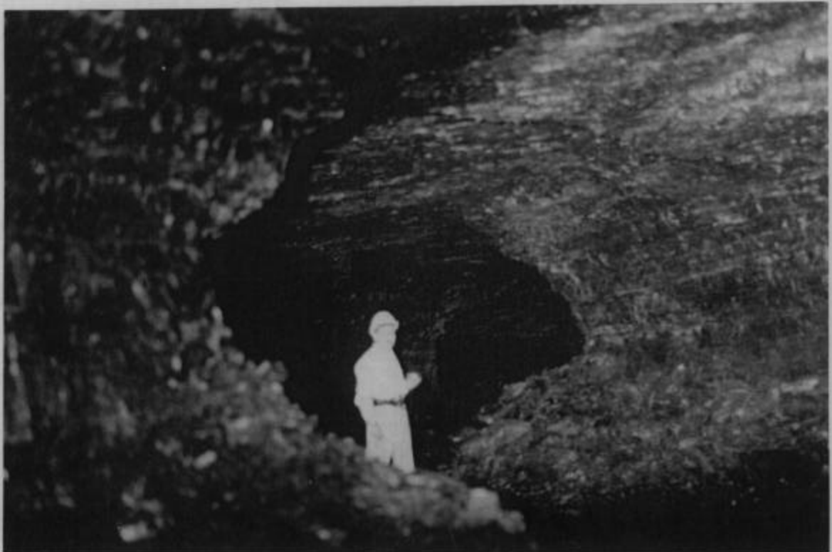
Figure 2.2. WIN (A) Rating 423 Poor. Showing Pillar Scaling Corners
