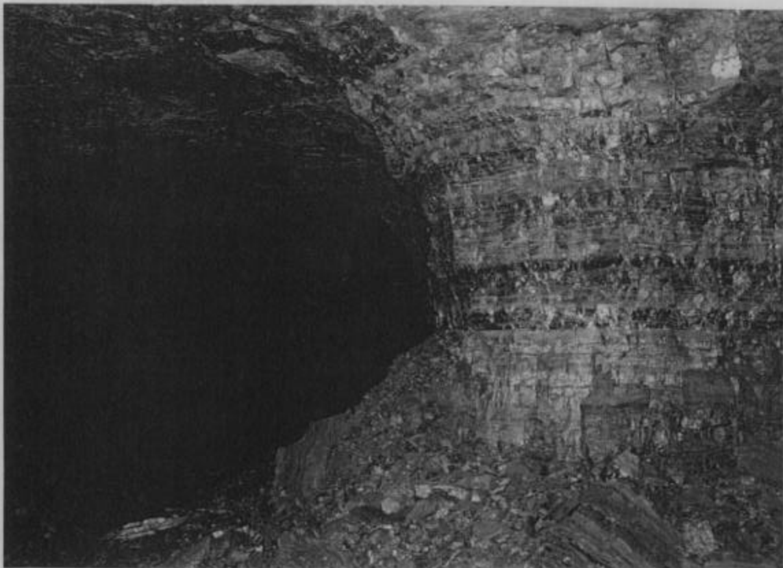
Figure 2.8. W2N (A) Rating 486 Fair. Scaling of Side and Corner
