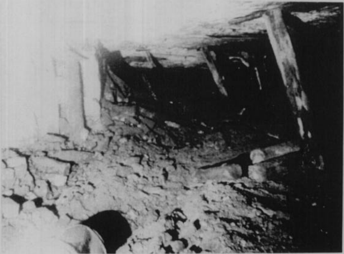
Figure 8.1. Floor Heave Natal and at an Australian Colliery
