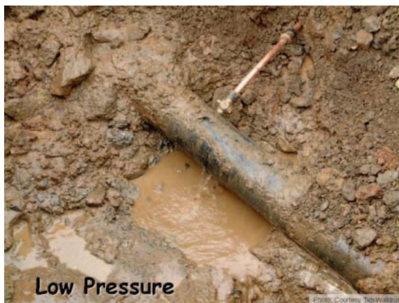
Figure 3: Typical burst water main at low and high pressure
