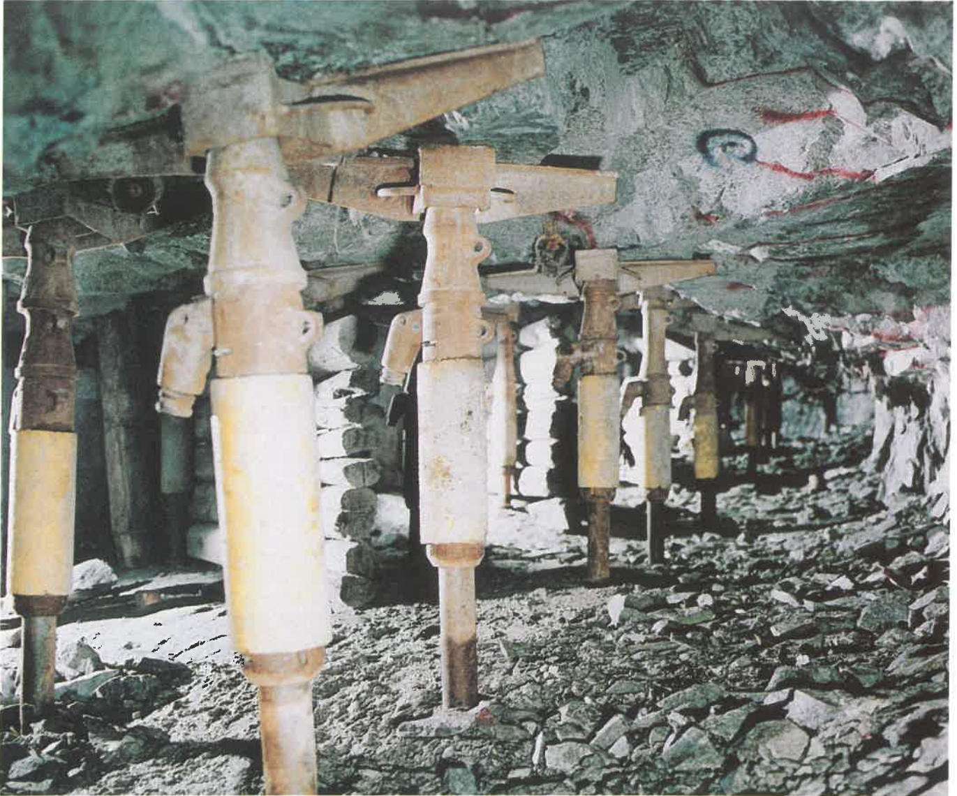
The lightweight 3 m/s rockburst prop and load spreader installed within a metre of the face in a deep gold mine. Note that the support comprises an integrated system of props, matching extension pieces and load spreader to ensure maximum coverage of geological and stress induced fractures, thus providing workers with maximum protection in the event of a fall of ground.
