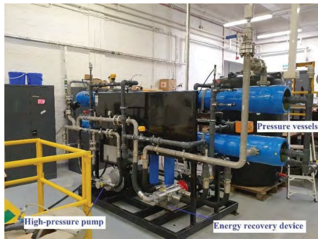
Fig. 1. RO unit installed at Aston University, UK [8].
