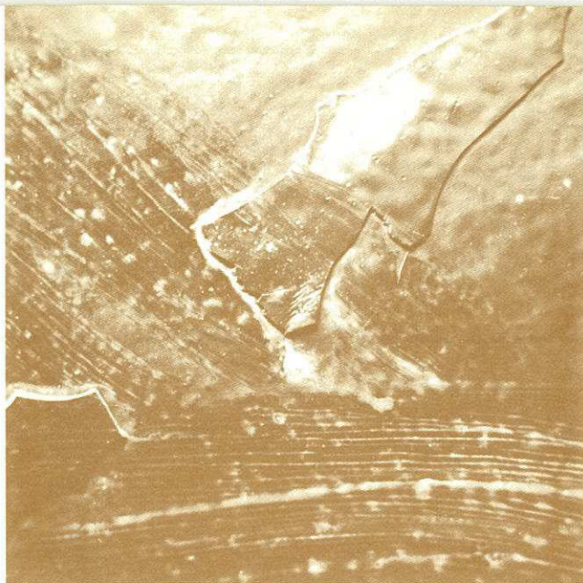
An example of delamination in epoxy tar coatings, which often occurs without apparent reason.
