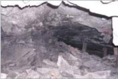
The CSIR has produced methodologies for assessing hazardous ground conditions on the UG2 when mining in the vicinity of Merensky Reef remnants
