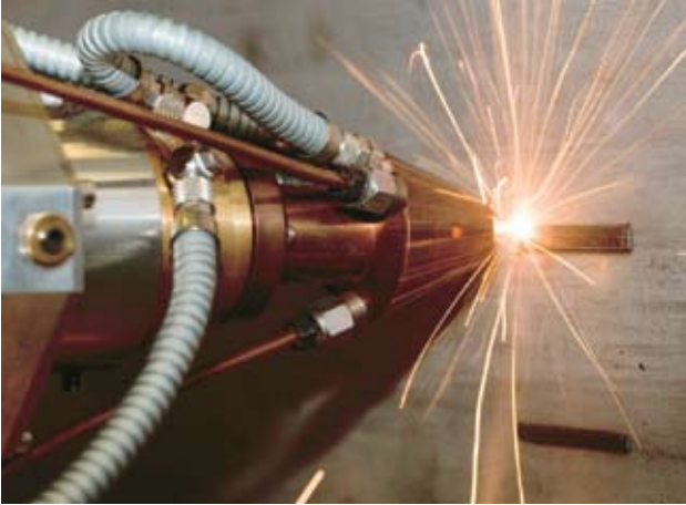
A demonstration of a world-first laser cladding system that offers a permanent solution to sealing leaks and repairing cracks at power stations.
