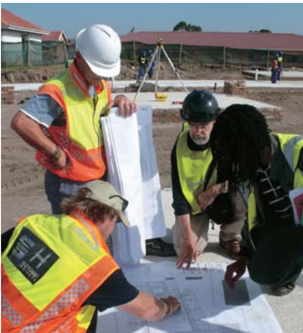
On location at the construction site of Catherine Booth Hospital in KwaZulu-Natal.
