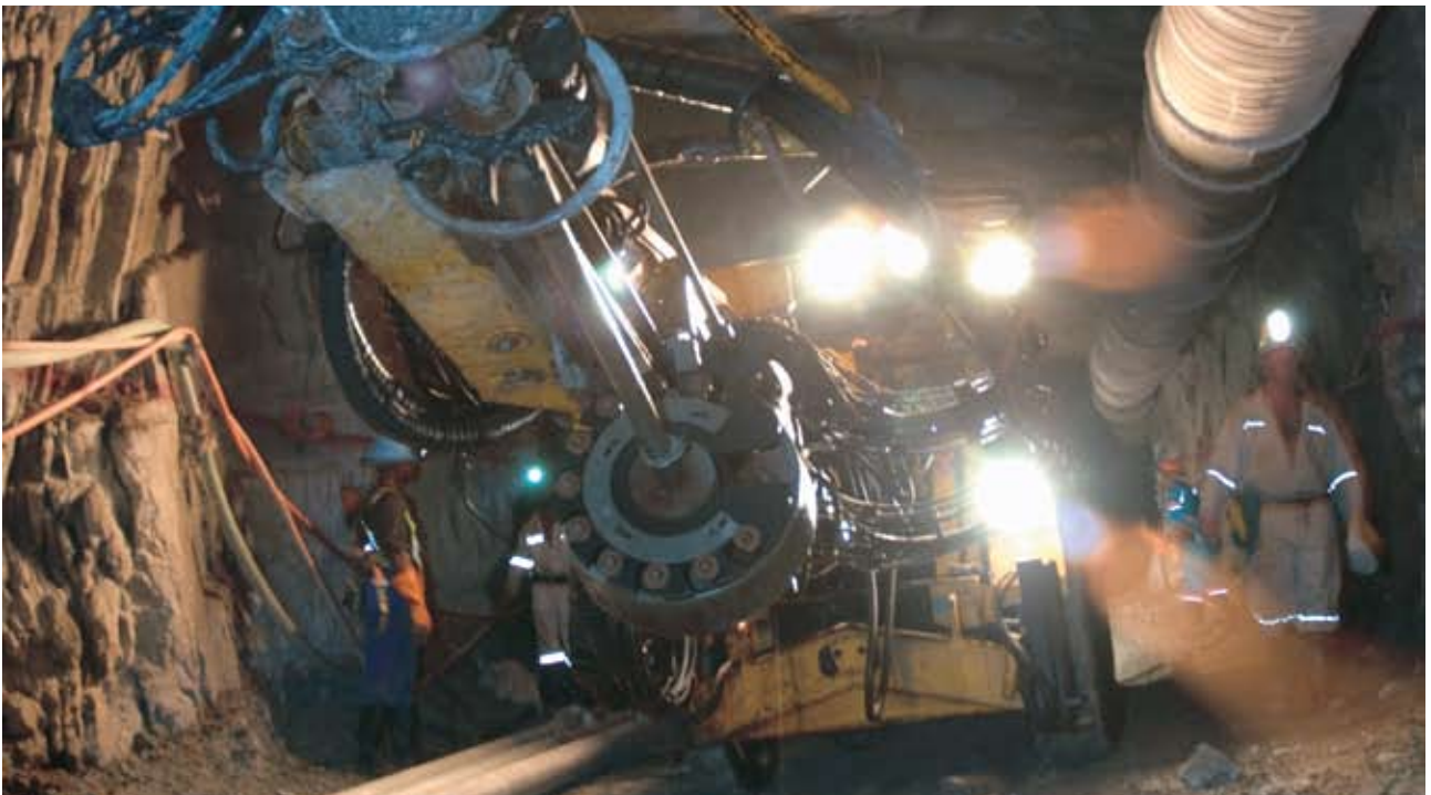
Rockfalls are a life-threatening reality in mines. An in-stope measurement system for underground sensing and communication, which also includes a number of sensors to gauge the condition of the roof, was developed by the CSIR.
