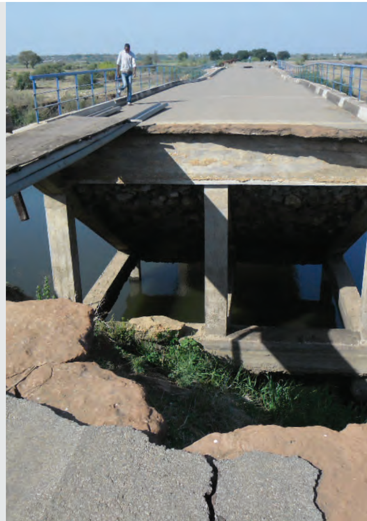
Undercutting and collapse of road embankment (left) and bridge abutment (right) due to flooding in the Gaza Province in Mozambique.
