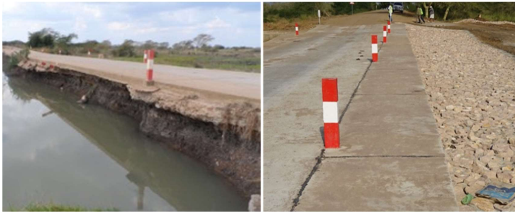
Figure 5 - Example site in Mozambique's Gaza Province, where the road has been adapted to address overtopping-induced erosion
