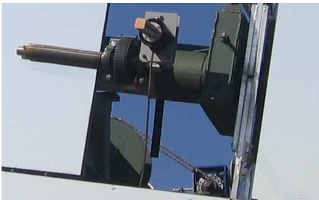
Figure 11: Close-up of solar tracker on 25 2 m heliostat torque tube.
