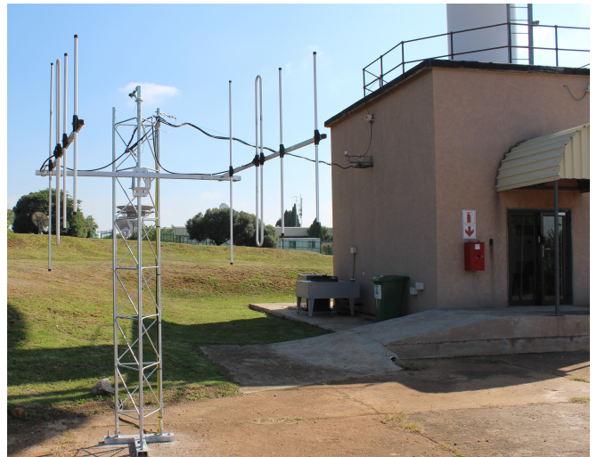
Fig. 1. Surveillance phased array.
