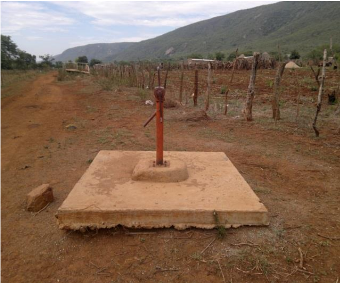
Figure 1: A non-functional borehole in Thambonkulu village, Mpumalanga
