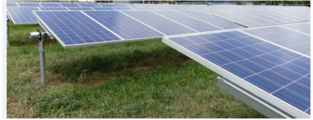
Figure 2: The 558 kWp single axis tracking solar PV plant
