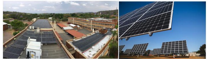
Figure 3: The rooftop and dual axis tracking PV plants at the CSIR in Pretoria
