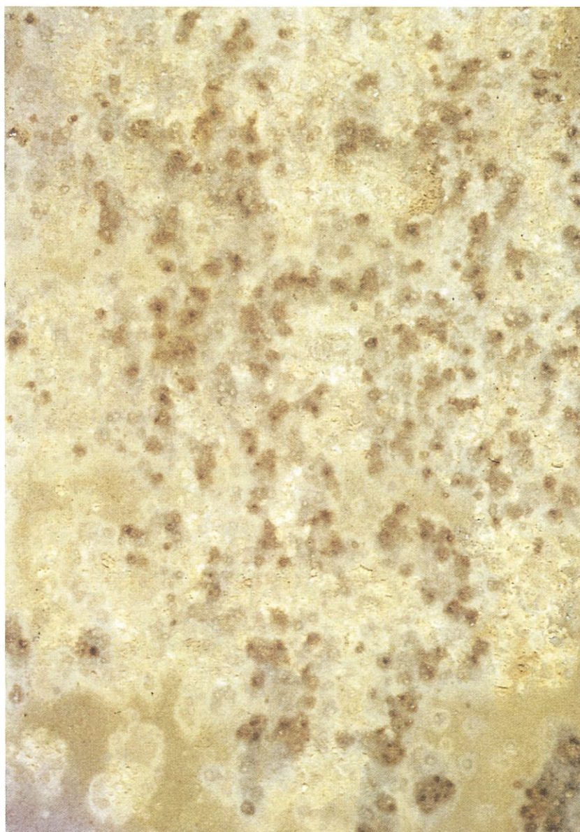
PLATE 13: Thermally Sprayed Aluminium applied to steel 25 years exposure at Walvis Bay (100 \mu\text{m} thickness, unsealed)
