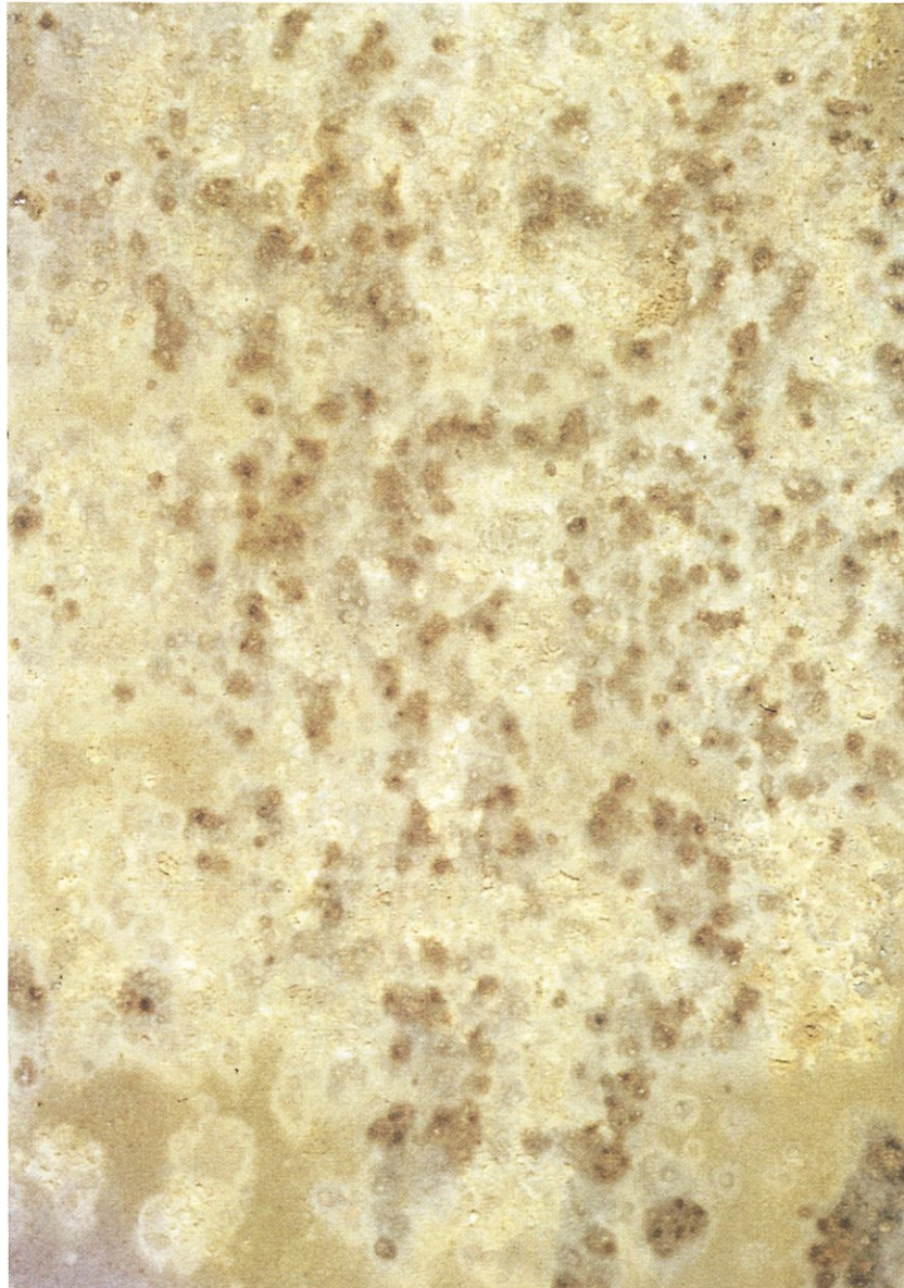
PLATE 13: Thermally Sprayed Aluminium applied to steel 25 years exposure at Walvis Bay (100 \mu\text{m} thickness, unsealed)
