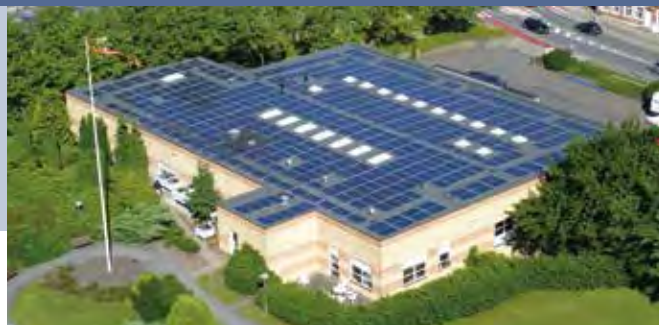
Fig. 2 - PV Solar Systems at the Regional Hospital in Viborg: A total of 280 kWh has been installed on 5 roof and area covering app. 10 % of the annual consumption at the hospital (Photo: Kenergy, Kenn H. B. Frederiksen).
