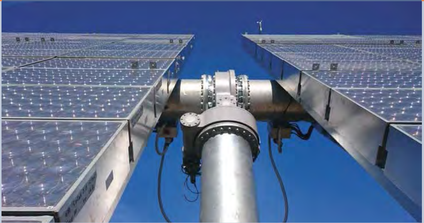
Fig. 3 - CPV plant installed at Monteveglio (BO) in the frame of the EU funded Ecosole project (Photo: Beghelli Becar).
