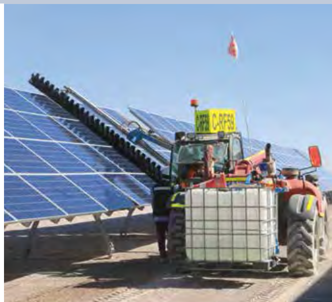
Fig. 5 - PV Cleaning System. 160 MW Finis Terrae PV Plant (ENEL Green Power) located at María Elena, Antofagasta Region, Chile.
