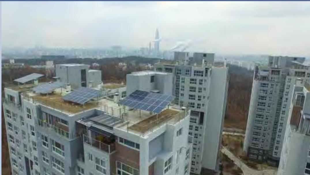
Fig. 3 - 142 kW roof mounted PV system installed by PV rental programme, Seoul, Korea.
