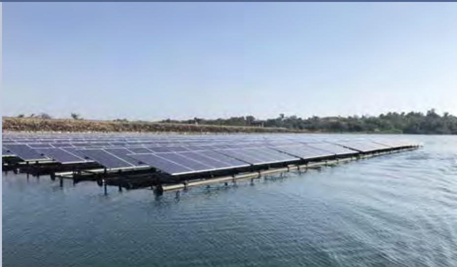
Fig. 2 - 250 kW Solar Floating Project by EGAT at Sirinthorn Dam, Ubon Ratchathani Province. This is a project for preparation and development of Solar Floating Systems in Thailand with the goal of continuing to target GW in 2021 (Photo: EGAT).
