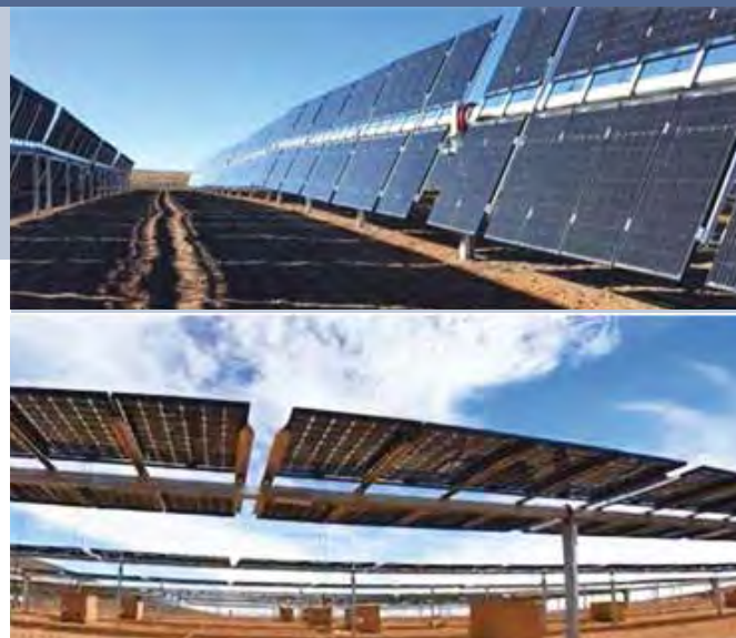
Fig. 2 - Bifacial modules Installed by EGP on one-axis sun trackers manufactured in Italy (Photo: ENEL Green Power).
