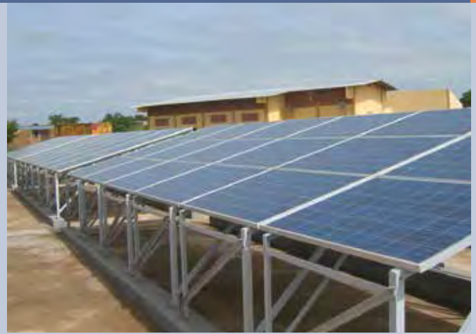
Fig. 7 - 216 kWc PV power plant, Mali, 2011 (Photo: IED France).
