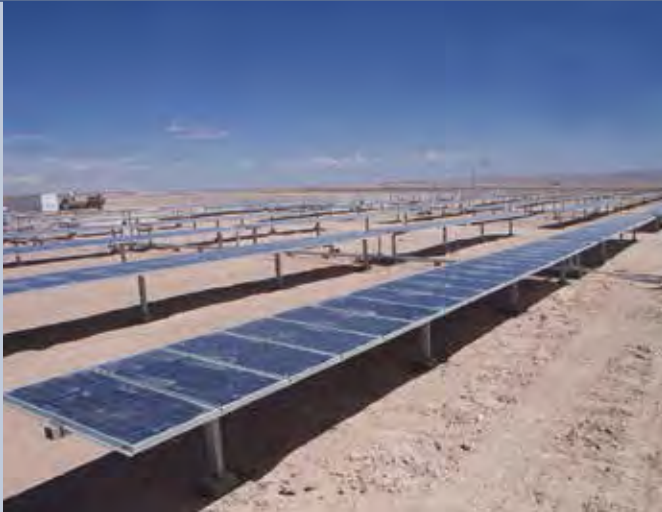
Fig. 1 - Calama Solar 3. This 1 MW power plant provides electricity to the industrial facilities of División Chuquicamata (the largest open-pit copper mine in the world).
