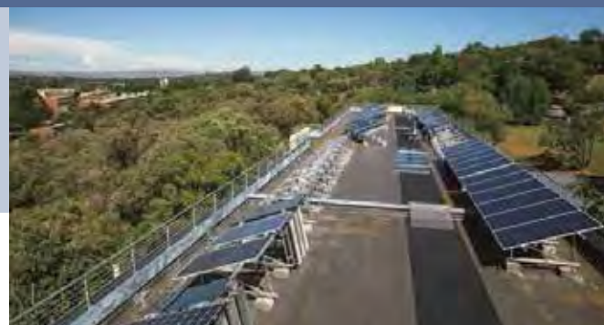
Fig. 2 - CSIR outdoor PV testing facility installed on the roof of the Energy Centre on the CSIR campus in Pretoria.
