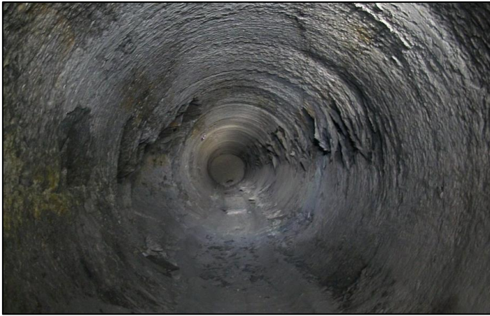
Figure 15. Photograph of hole 17 taken from the upper reef drive, showing spalling on the western (right) sidewall that occurred only after the hole 18 was drilled.
