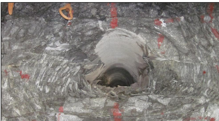
Figure 12. Photograph of exposed reef raise face, revealing extensive fracturing beyond the extent of breakout around the hole.
