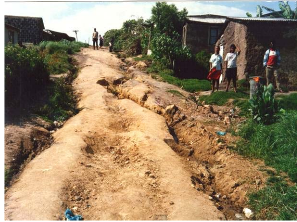
Figure 2: Poor road conditions as a result of a lack of maintenance could negatively impact on the safety of commuters.
