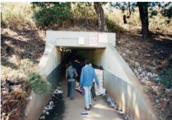
Figure 5: This dark, narrow subway does not feel safe and provides ideal settings for pedestrians to be victimised.
